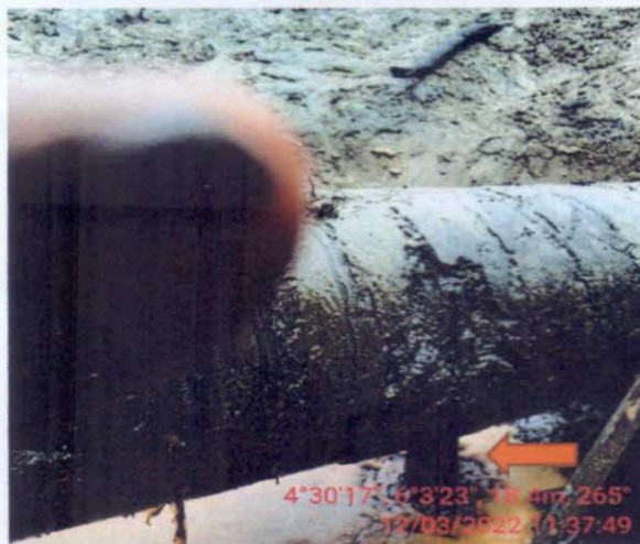
FIG. 1: SHOWING CORROSION POINT AT 6 O' CLOCK POSITION.
